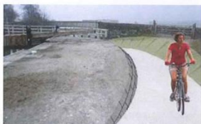
Regrade slope as much as possible to improve gradient, needs further talks with CRT, gate position is new and could be relocated to right of pedestrian gate giving more space for regrading of slope.
