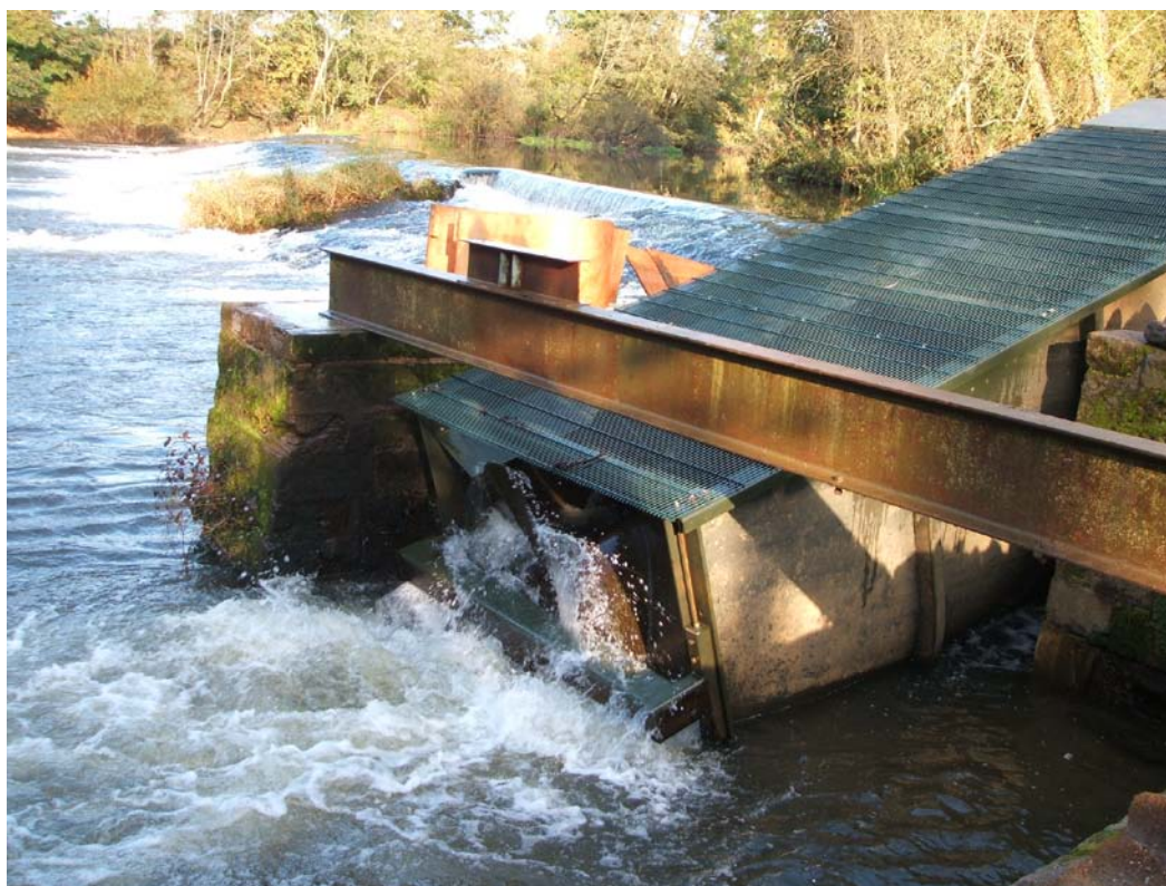
Archimedes screw at Howsham Mill
