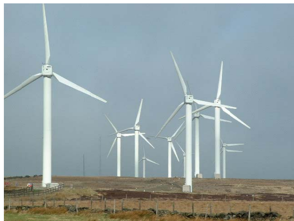
Figure 19 The 9 MW, 23 turbine, Ovenden Moor Wind Farm in Calderdale. This wind farm has been operational since 1993 and an application has been submitted to planning for repowering of the site with larger turbines. (Source: Nigel Homer, March 2005, retrieved from Wikimedia website, accessed November 2010)
