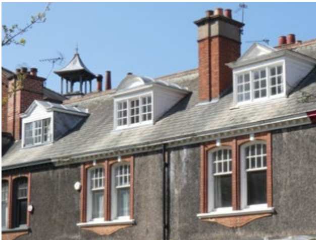
4.3 Slated roof with dormers to Edwardian property close to the Abbey (Insall)
