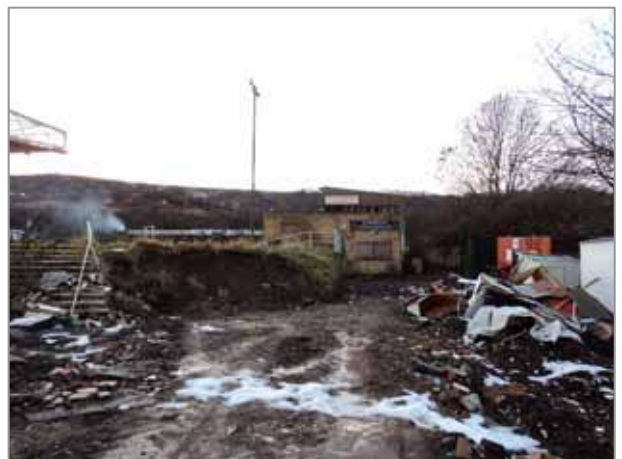
Image 12: McCain Stadium – Dug up driveway from main entrance
