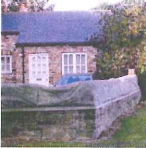
Temporary flood defences in Selby
