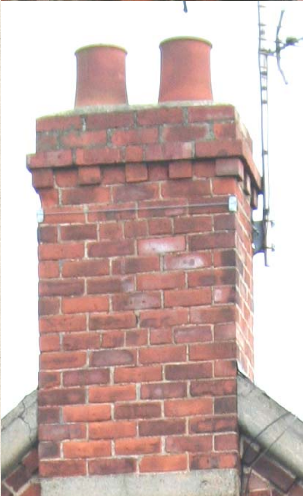
Left: Gable roof with round window Top: Deep red pan tile roof covering Above Tall decorative chimney
