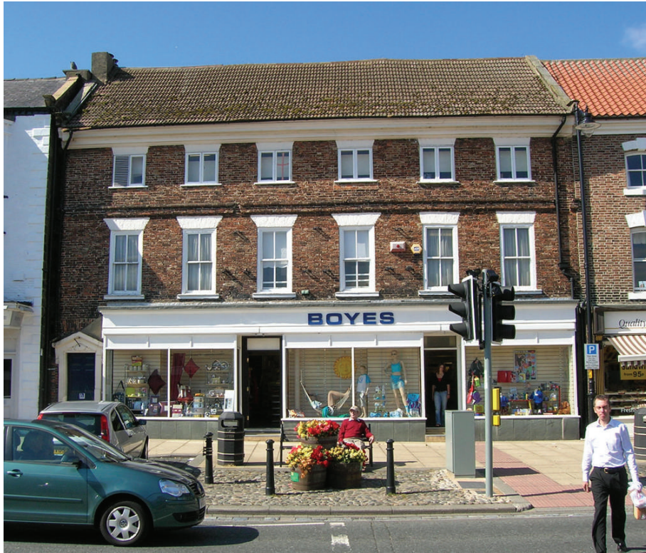
Figure 11: There is no visual support to the upper floors from this 1960's shopfront.
