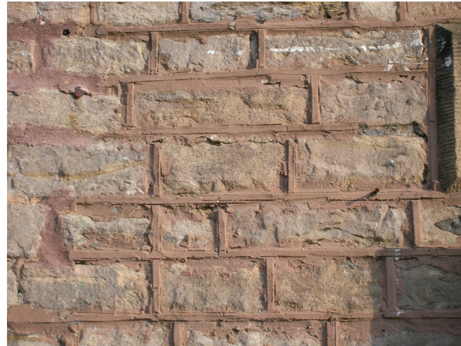
Figure 23: Inappropriate cement mortar finished to a strap profile not only adversely affects the appearance of the building but also will lead to accelerated erosion of the stone.
