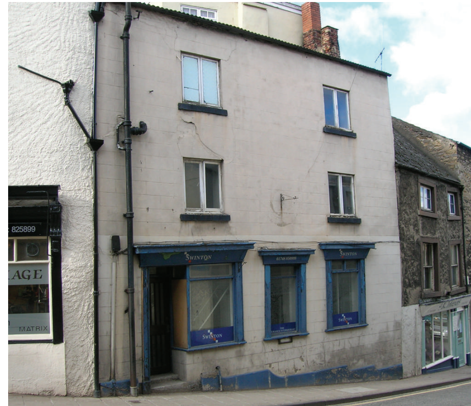
Figure 25: Inappropriate cement render has cracked and will allow moisture to penetrate into the building.
