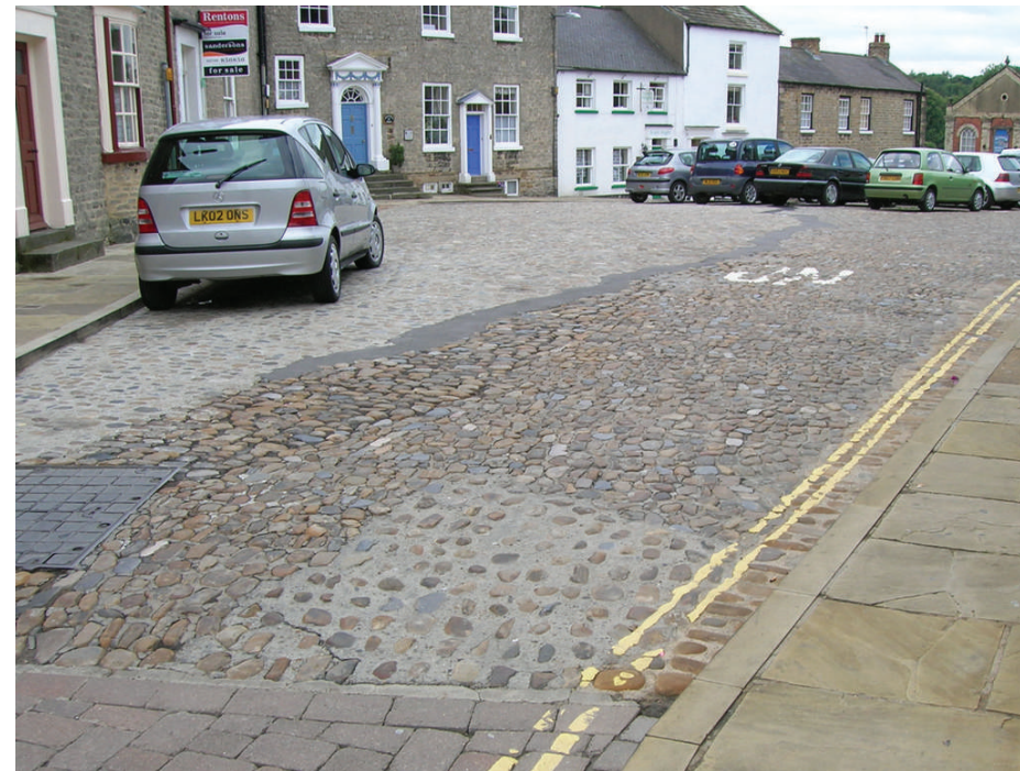
Figure 31: Modern repairs made to the historic street surface.
