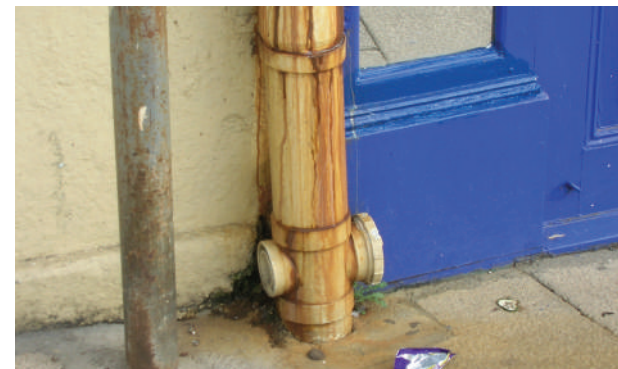
Figure 22: Base of original cast iron rainwater pipe repaired with inappropriate plastic section.
