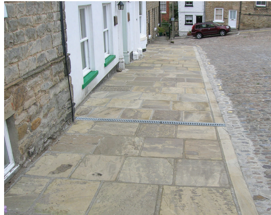
Figure 32: Footpath repaired with local materials. The kerb line provides definition between the road and footpath.
