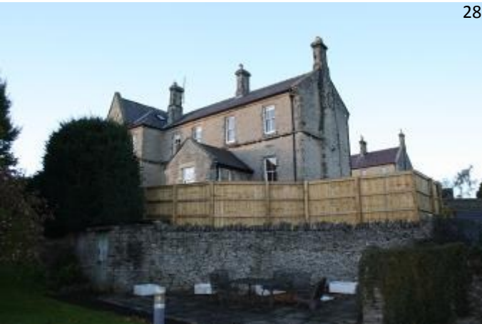
These appear to be contemporary to the original building and as they appear on the 1895 OS map they are considered to be original features. Their construction detail and regard for other elements of the main building such as the prominent string course and window spacing also suggest they formed part of the original building. It is noted that the string course only extends as far as the projecting chimneys at each gable end, (photo 28) the expense of decorative sawn stone being spared away from the principal elevation of the building.
