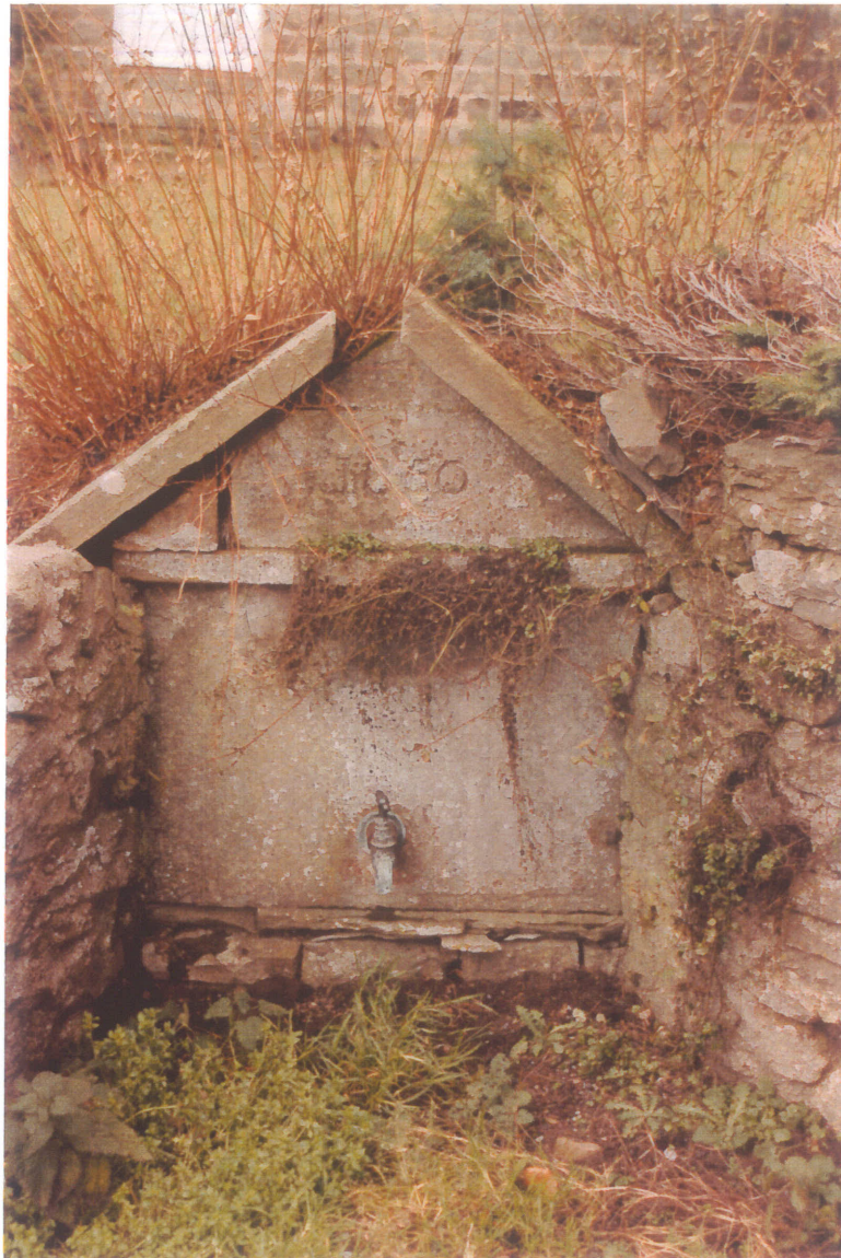
Water pump, dated 1850, largely intact but in need of some repair
