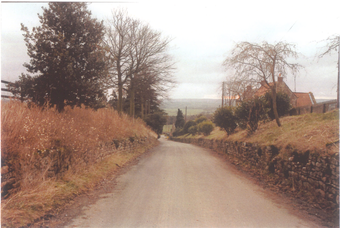
walls within the 'cutting' are important to the overall character of the village, but are in need of repair
