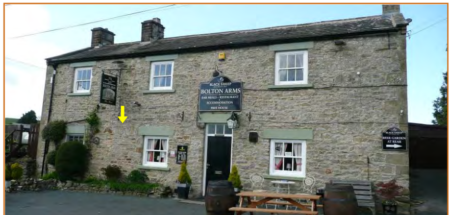
Figure 29: The Bolton Arms pub; the arrow points to a blocked former door with a flat-arched head made of voussoirs; also note the green painted lintels indicative of the former MoD ownership (photo © Gaby Rose, YDNPA, 2017)
