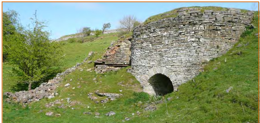
Figure 42: Lime kiln at Downholme Quarry, with adjoining retaining wall visible to the left (photo © Gaby Rose, YDNPA, 2017)
