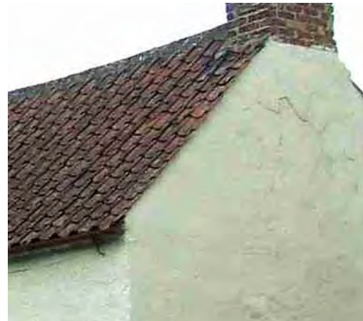
Render is widely used in Wath to cover brickwork, cobble walling, and, in some instances, stone.
