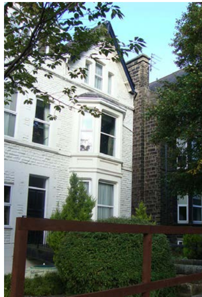
This photo demonstrates the dramatic effect that painting previously exposed stonework can have on the appearance of a building.
