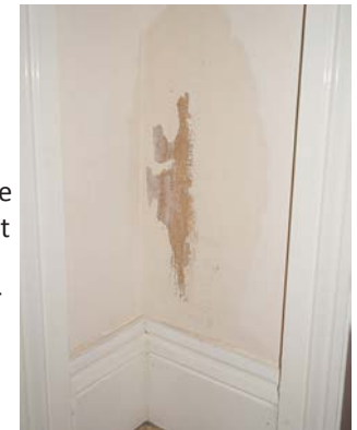
Damp problems within an historic building that have occurred since the installation of a damp proof course – this will have introduced impermeability with the wall fabric.
