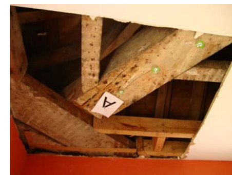
A carefully considered structural assessment being carried out to historic timberwork in order to inform a repair scheme.
