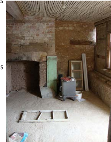
Historic fabric, including internal plasterwork, should be retained and repaired wherever possible. The wholesale stripping out of interiors, as seen here, is not acceptable.
