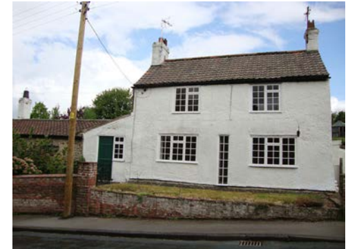
Inappropriate re-fenestration, together with alterations to the openings, has harmed the character and appearance of this non-designated, traditional cottage.
