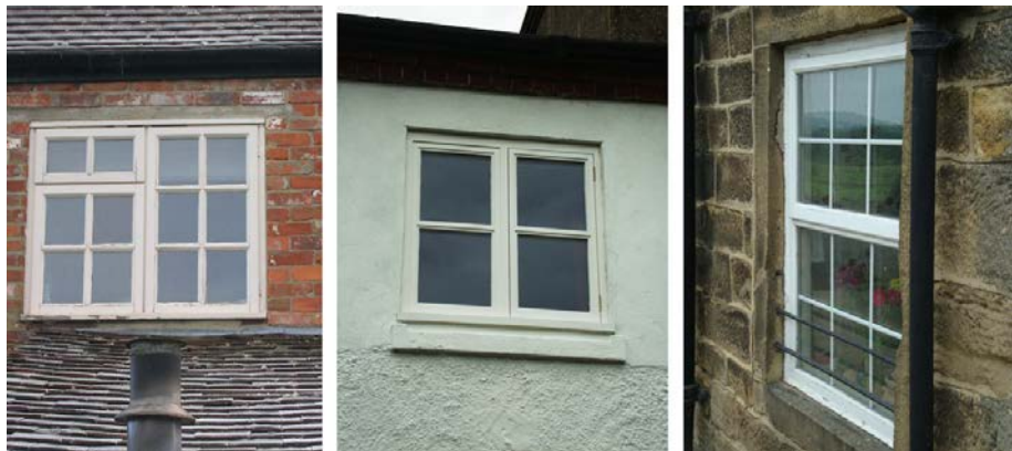
Inappropriate window types: storm proof profile and a top opening light/double glazed window with non-traditional glazing bar and with a poor relationship to the historic cill/internal glazing bar within the double glazing unit.
