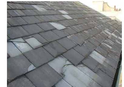
Poor quality slates laid instead of better quality Welsh slate – after only five years, severe lamination has occurred and replacement is required – a false economy.
