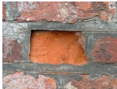
Inappropriate re-pointing carried out with cement mortar has accelerated decay and disfigured the brickwork.
