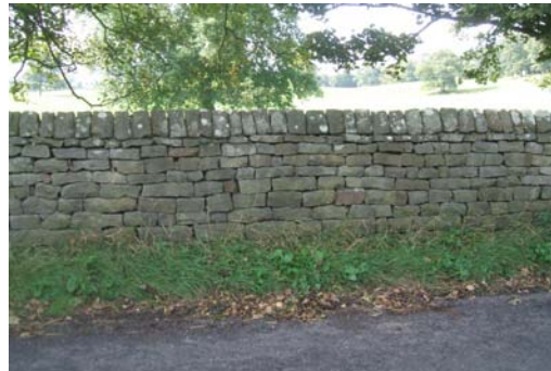
Pennine dry stone walling is by far the most common boundary feature in the Conservation Area.
