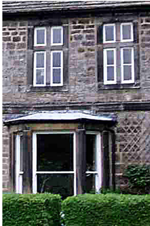
Weston Grange: one elevation, two different eras, two different window types. At first floor the mullioned and transomed casement windows are original to this late seventeenth century building. The large single paned sash windows were inserted in 1890.
