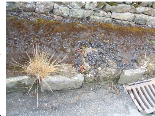
Kerb repairs needed.
