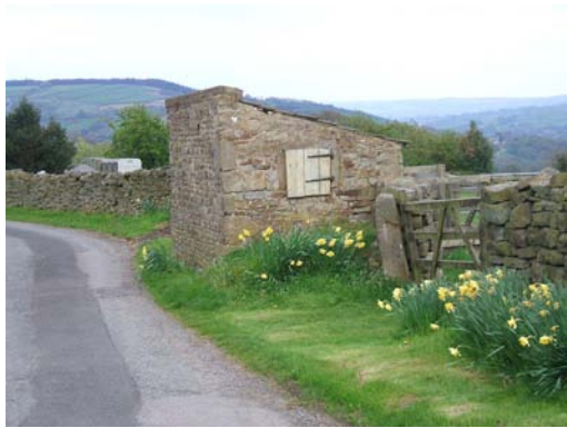
Outbuilding on south side of Back Lane at the top of a strip field.
