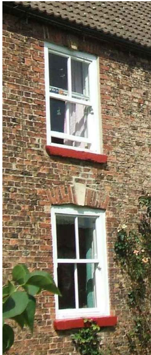
Window openings with a gently cambered head (lower) and a flat gauged brick arch head (upper) at Staveley Farm
