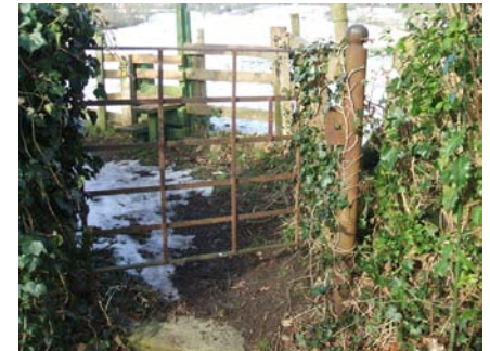
Gate needing repair at Spring Lane
