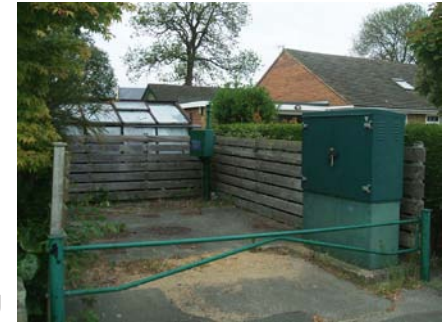
Gas valve house in need of screening
