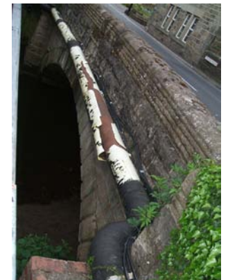
Disfigurement of Pannal Bridge
