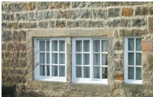
Window detail at 25 Main Street (unusually two Yorkshire sliding sash windows linked together).
