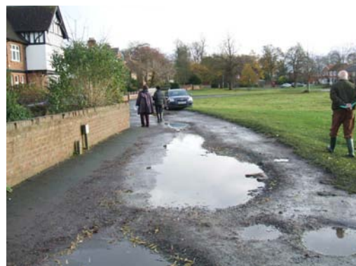
Poor surfacing of tracks and erosion at the edges of the green.
