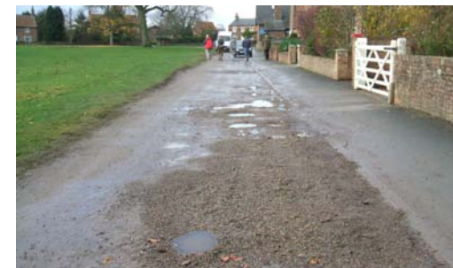
Tracks around the green are in need of resurfacing.
