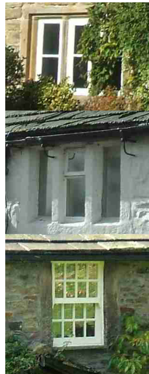
Windows through the ages. Top: double chamfer mullion windows in chamfered reveals. Middle: an eighteenth century mullioned opening with square mullions and square reveals. Bottom: a sash window.
