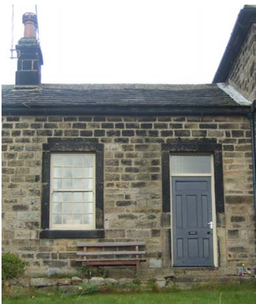
Stone slate, stone walling, lime mortar and timber gutters, windows and doors are the most commonly used material in the Conservation Area.
