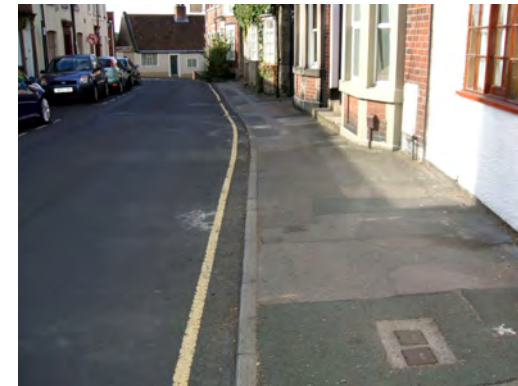
Patchy bitmac pavement on Finkle Street.
