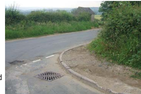
Localised vehicle erosion of grass verges.
