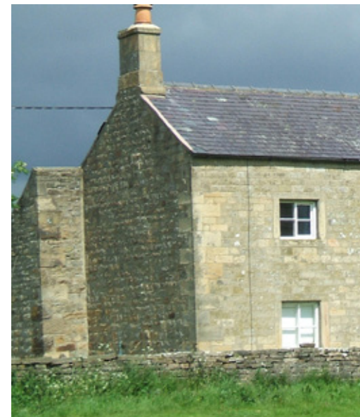
The formal front elevation has smoothed stone, the less important side elevation is faced with less dressed stonework
