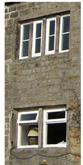
An example of an eighteenth century mullioned window (top) and the same opening, but with two of the mullions removed (bottom) to create large openings which are suitable for sash windows.
