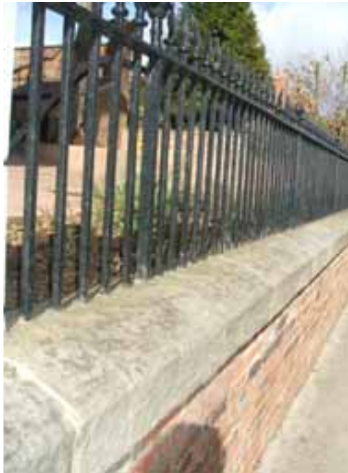
Railings atop stone copings on a brick wall bound a property on Horsefair.
