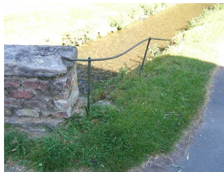
If not carefully monitored simple elements can be lost over time.
