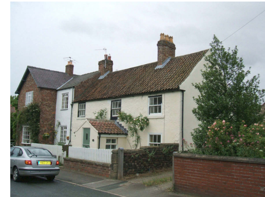
Traditional timber sliding sash windows in the foreground and replacement modern casements in the adjoining property, showing how character can be eroded gradually through the loss of traditional detailing.
