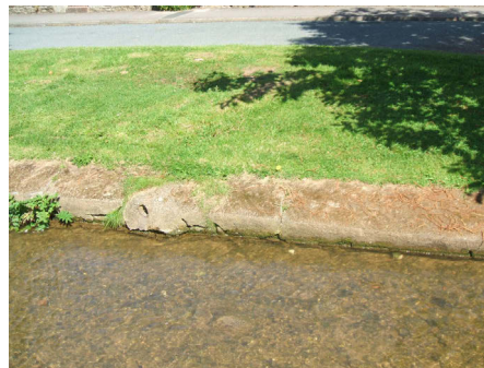
Inappropriate concrete infill has taken the place of stone.
