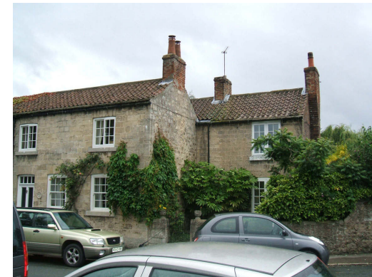
Pantile roof with gable chimney not expressed externally. This roof has a simple clipped eaves.
