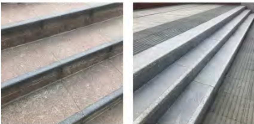
Picture 4.1 Steps can be hazardous and should incorporate nosings in a contrasting colour and hazard paving at the top and bottom of flights
