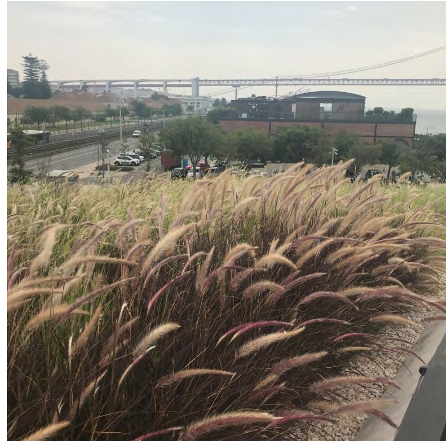
Figure 12.11 An extensive green roof planted with ornamental grasses
