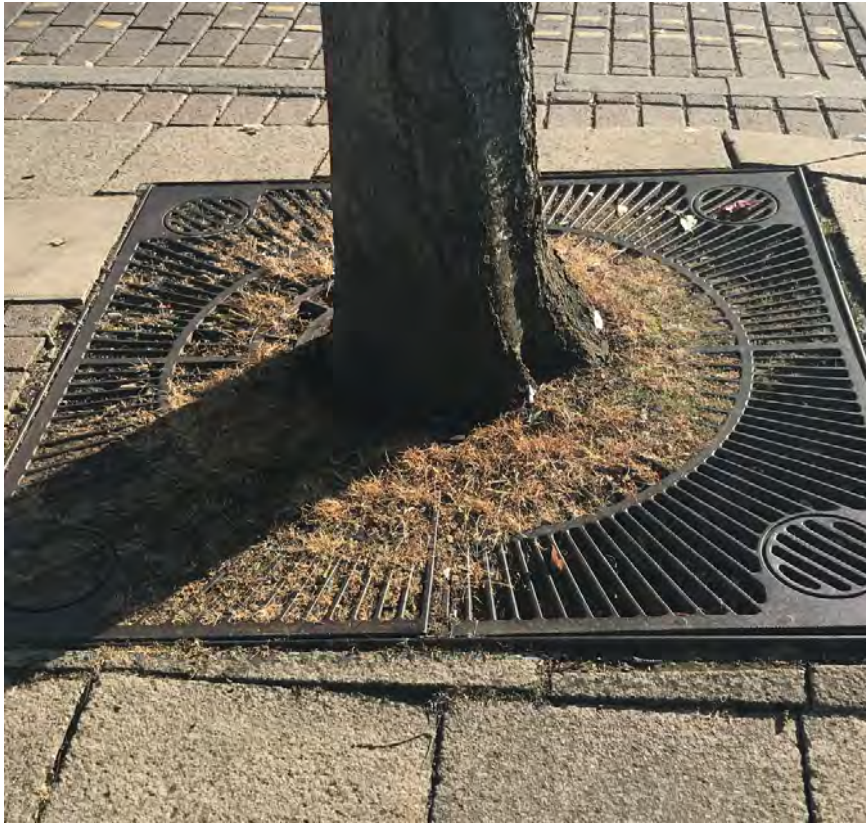
Figure 8.5 Tree grilles often present maintenance problems causing trip hazards, filling with soil or rubbish and require removal when the tree outgrows them
