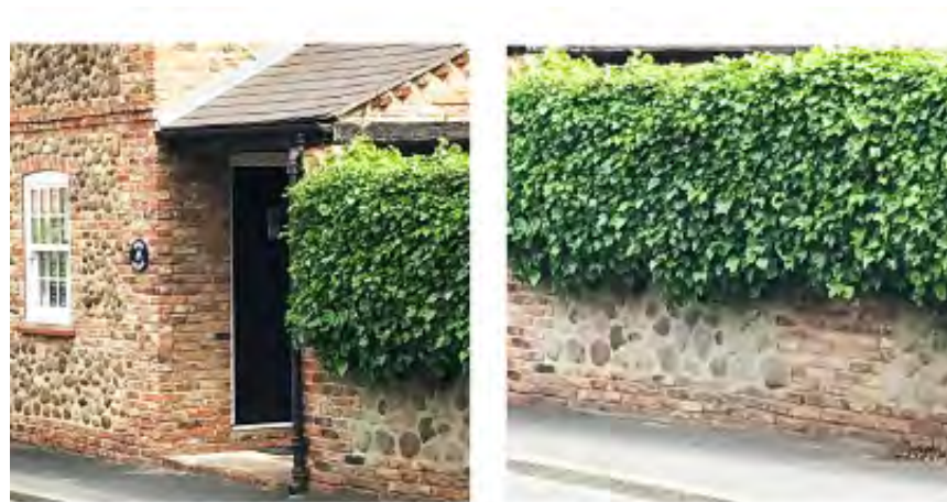
Figure 5.7 Example of traditional brick walls with panels of field stones in Green Hammerton
