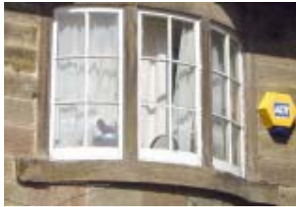
Intrusive and poorly located burglar alarm, Chantry House Gallery.
