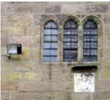
Insensitive type and positioning of floodlighting unit, Castle Gatehouse.
