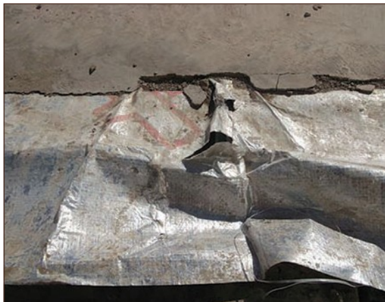
Figure A4.54 Gas membrane damage/tearing at edge of ground floor slab screed layer where it was left exposed to elements for period of time (courtesy NHBC)
