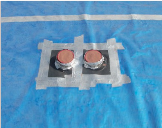
Figure A4.27 Top hats placed around service entries secured with jubilee clip seals. Top hats secured to gas membrane with double sided butyl tape (courtesy Hydrock)
