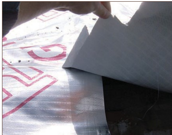
Figure A4.76 No double sided tape used in joints (courtesy Smith Grant)
