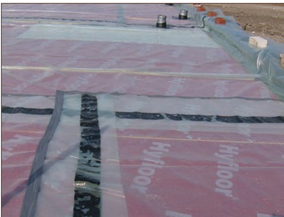
Figure A4.65 Wrinkling of gas membrane over joint has resulted in gaps (only visible due to the use of a transparent gas membrane) and the secondary seal uses ordinary gaffer tape rather than a proprietary product (courtesy Smith Grant)
