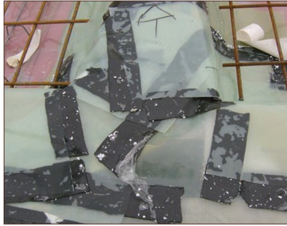
Figure A4.68 A pre-formed corner unit would have been preferable. The installer could not produce sufficient quality despite the amount of tape applied (courtesy Smith Grant)
