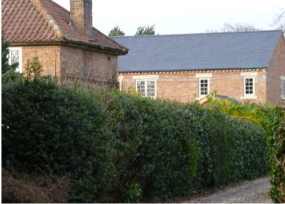
Unsuitable roofing material in Roecliffe Village
