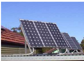
Solar photovoltaic panels (Solar PV) that produce electricity.
