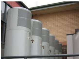
Water source heat pumps
