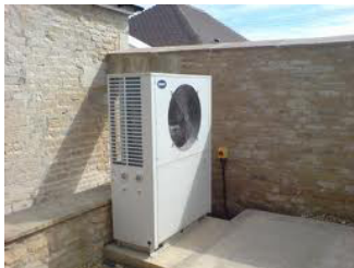
Air source heat pumps
