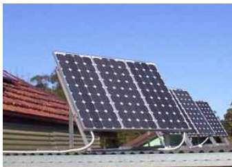
Solar photovoltaic panels (Solar PV) that produce electricity.
