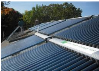
Solar hot water collectors that, as the name suggests, heat water.
