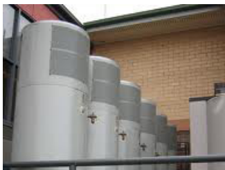
Water source heat pumps
