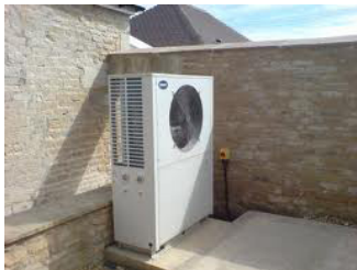
Air source heat pumps
