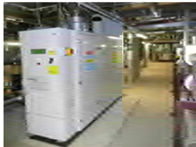
Figure 8: Energ100kWth, 70kwe CHP plant, installed at Highbury Stadium redevelopment, London. The 70 kWe electrical output feeds the landlord's supply and provides a base load for communal services. All new homes are on a district heating system; the heating and hot water is controlled through a heat interface unit inside each property (Source: AECOM, 2009).
