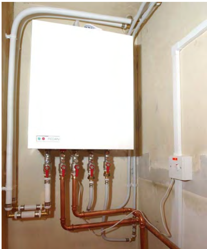
Figure 10: A heat exchanger inside one of the flats connected to the Aberdeen district heating network. Equipment is similar in size to a gas boiler (Source: Aberdeen City Council: a case study of community heating CE65, Energy Saving Trust, October 2003)
