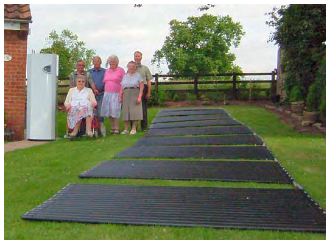
Figure 17 Ground panels laid out prior to ground work commencing on installation of ground source heat pumps (Source: Copt Hewick Ground Source Heat Pump Project Case Study 2007, Ryedale Energy Conservation Group)
