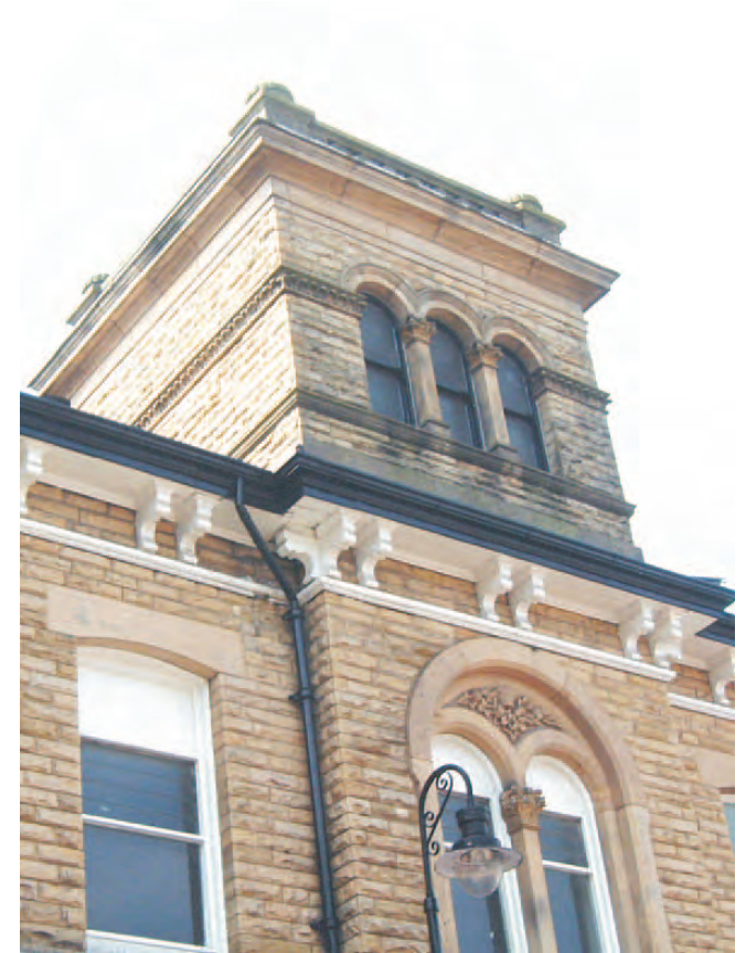
Hewn, dressed and carved stone details. Small course height at high level.
