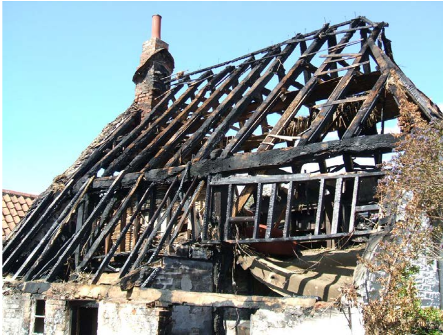
Fire damage at the Thatch Cottage, Long Marston.
