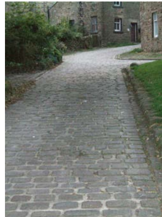
Stone setts laid across slope, gutter formed of setts laid down slope, random stone blocks forming kerb to grass verge.
