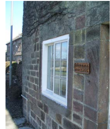
Slim double glazing units held in place with putty.
