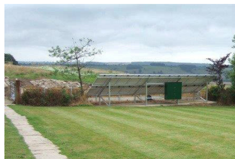
Ground mounted solar panels.
