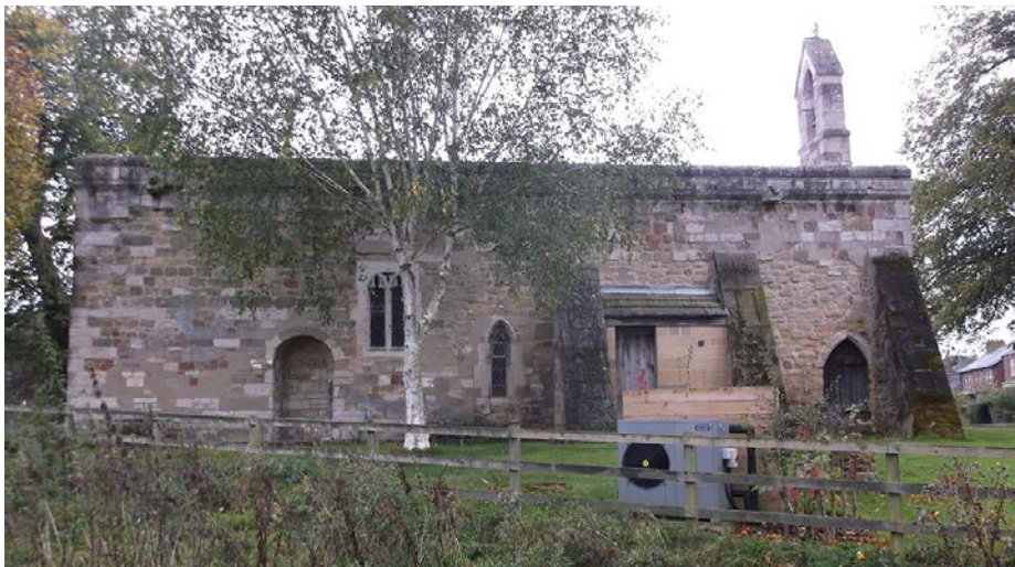
Recently installed air source heat pump at Chapel of the Hospital of St Mary Magdalene, Ripon, a grade I listed building.
