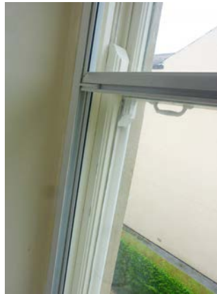
Secondary glazing installed on the inner face of a traditional vertical sliding sash window. Note that the secondary glazing lines through with the meeting rail of the sash window and is not therefore visible externally.
