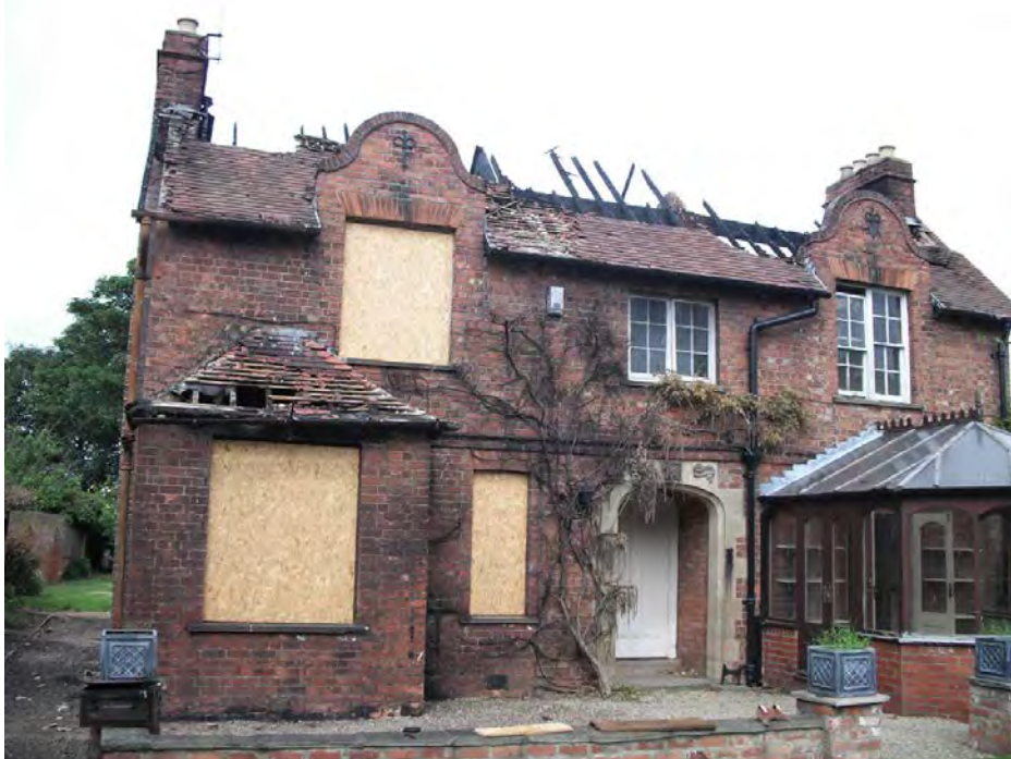
Fire damage at Priests' House, Allerton Mauleverer Estate.
